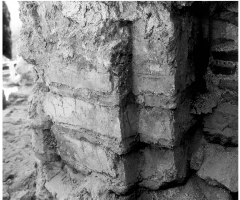
7b) Older photo of the middle dome taken during the 80s work also showing the recessed-brick technique (now covered by the lead sheet roof)
