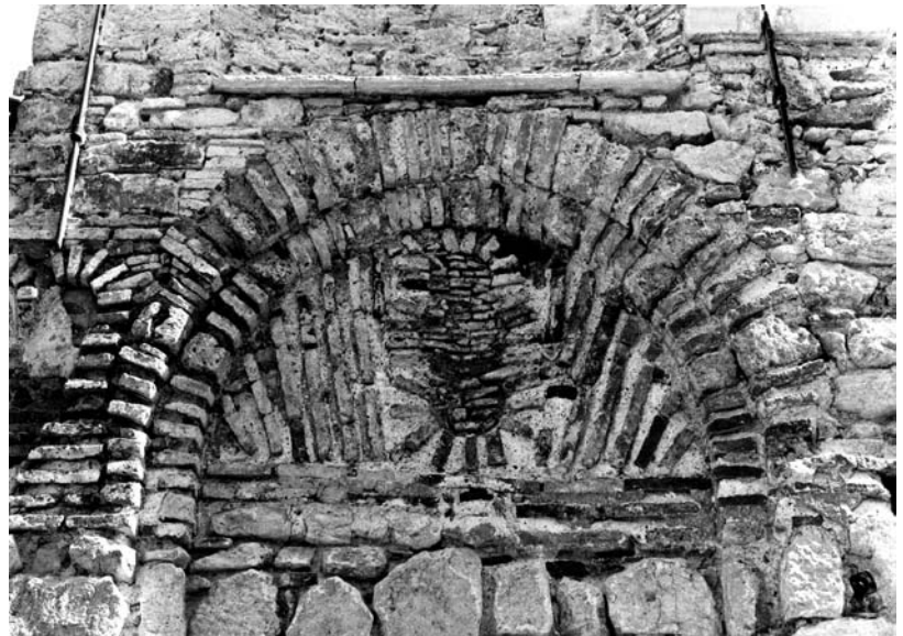
5b) South façade west arch (courtesy of the 3 rd Ephorate of Byzantine Antiquities)
