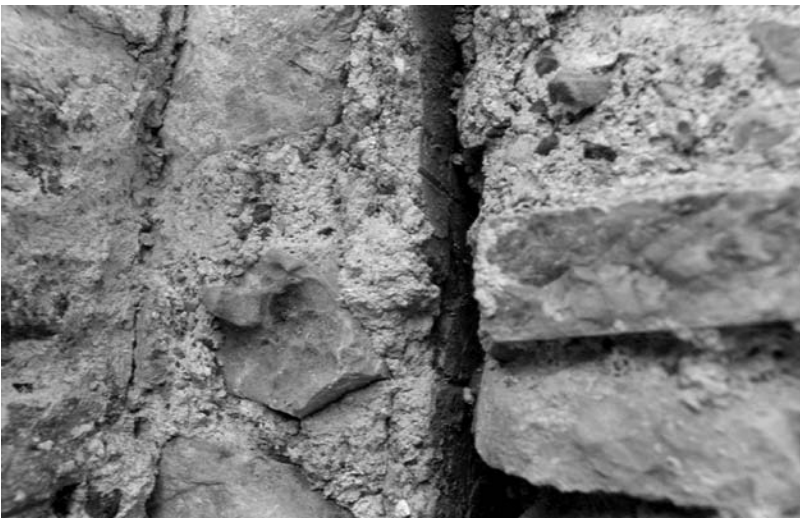
6b) View of the junction between exonarthex and annex. Pink plaster finish can be seen in the gap between the two buildings
